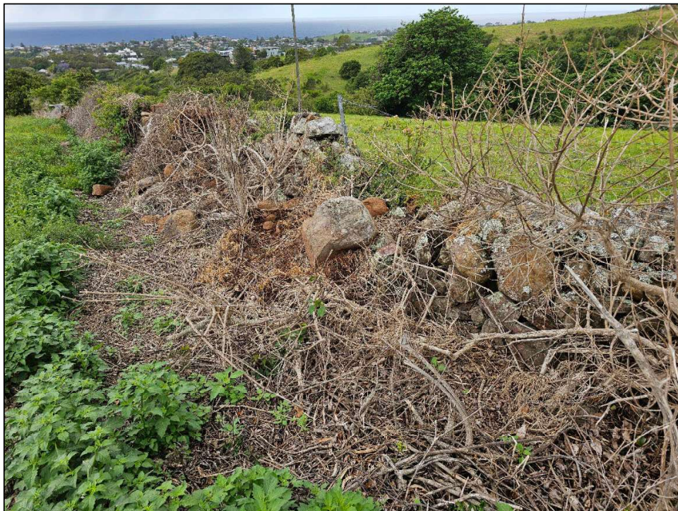
Photo 2 – Typical dilapidated section of dry stone wall recommended for restoration through removal of vegetation and reconstruction using traditional materials and techniques.
